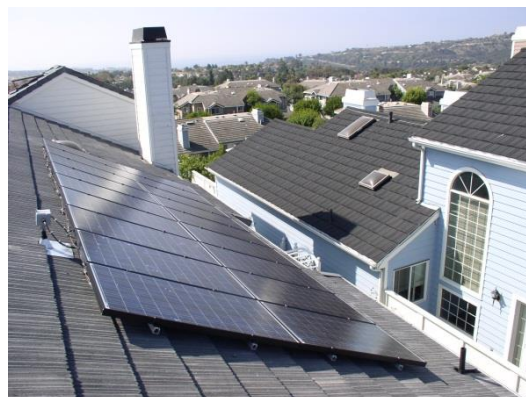
Figure 5.2: PV roofing (Source: Suntappers Website)
