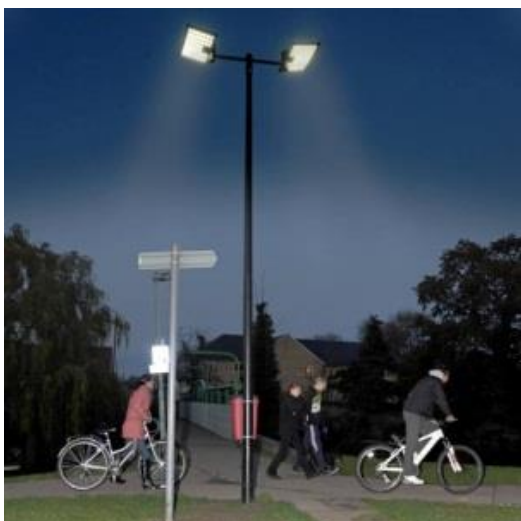
Figure 8.7: Streetlights illuminating walkways
