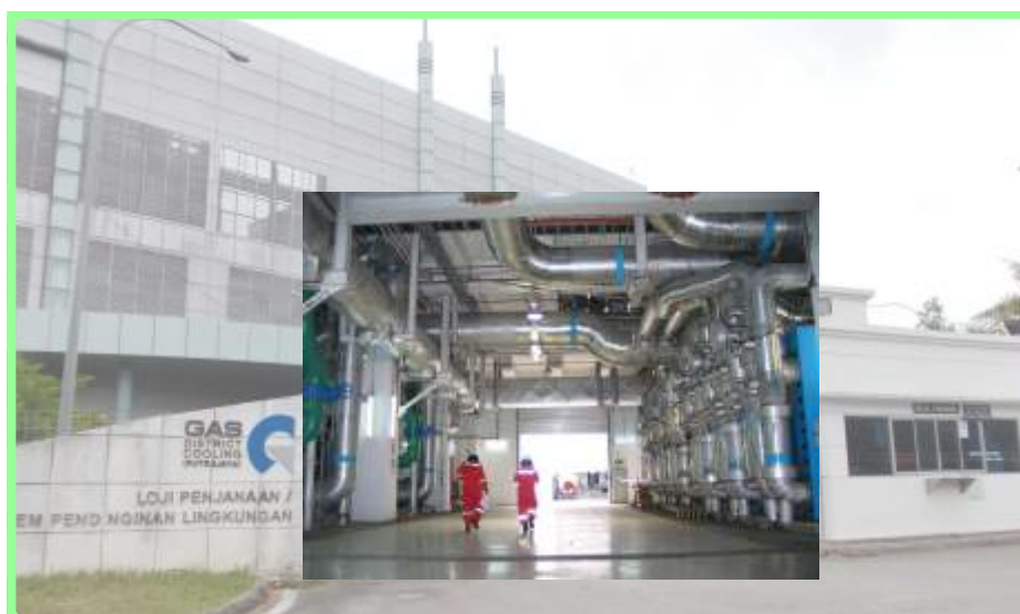
Gas District Cooling Plant
